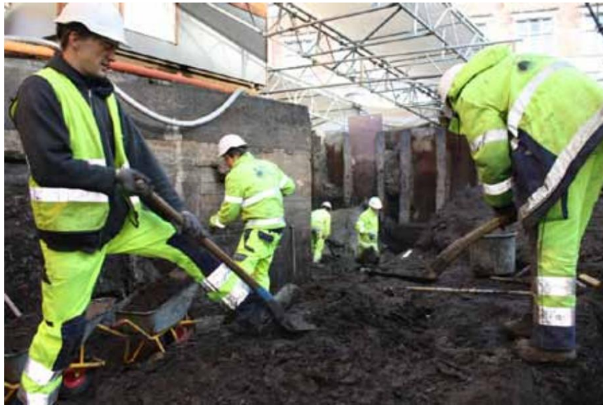
Fig-2 Town Hall Square below archaeological excavation. Note the dark "soil" that is dug in. It is in layers like these that the organic material thrives in, as the conditions are very moist.
